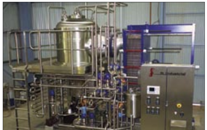
CT-9 for tea and coffee extract installed 2003
