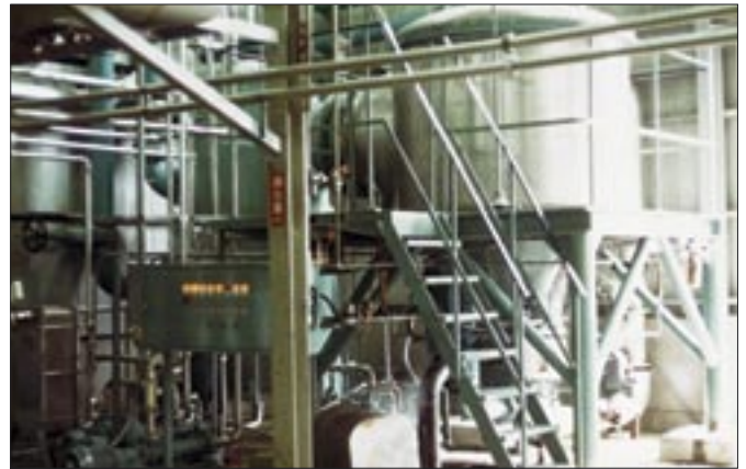
CT-9 in a Pharmaceutical plant installed 1970
