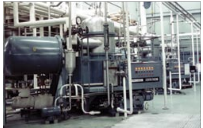
Three CT-6 plants for the recovery of solvent installed 1974.
